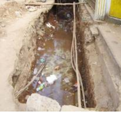
Storm water drain coverage of only 20%
